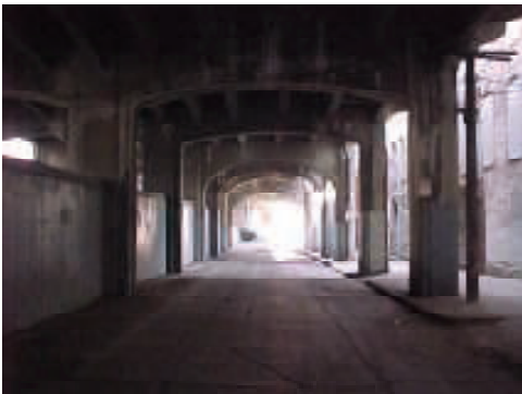
The road and sidewalk under the Eighth Street Viaduct is intimidating and dark.
